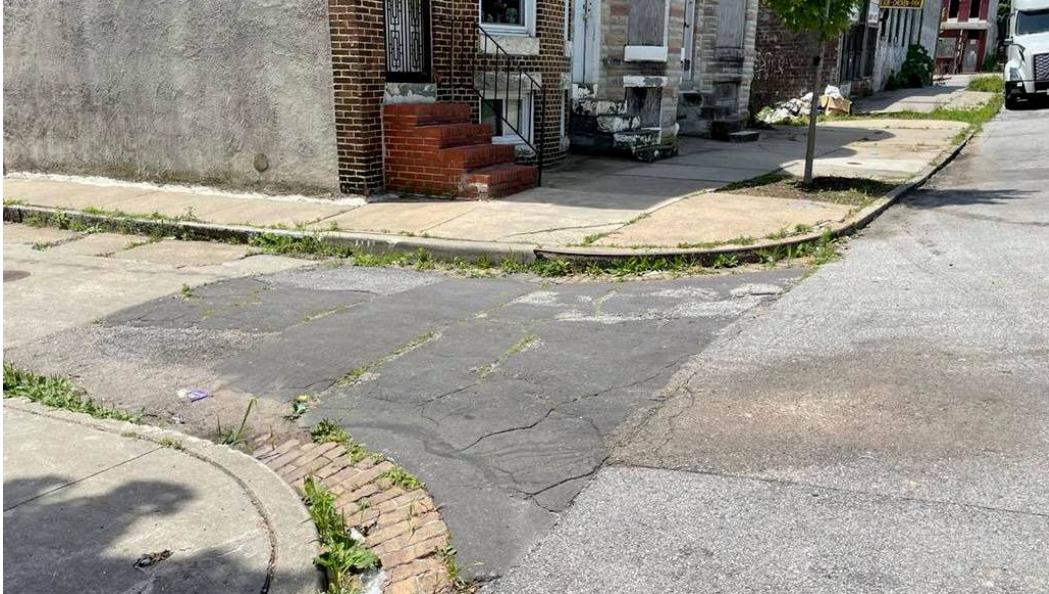
Curb ramp were never installed at the Bruce Street intersection with Westwood Avenue in West Baltimore. (Fern Shen)
